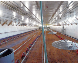
Gas heating equipment
