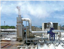
Waste steam recovery systems
